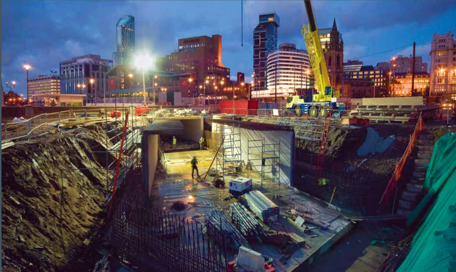
Work continues on Liverpool Canal Link, against the background of the Commercial District, 2007
