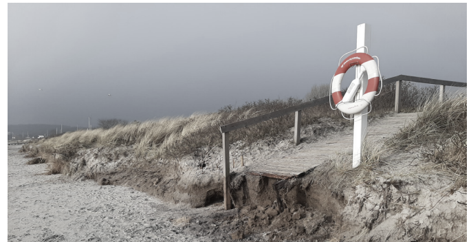
Photo: Coastal flooding has eroded the dike and staircase south of Aarhus. December 2023.
